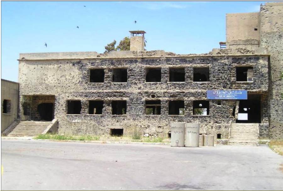
Figure 25: Destroyed hospital in Qunaytra.
